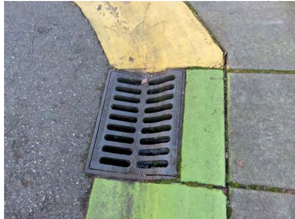
Typical Storm Drain
