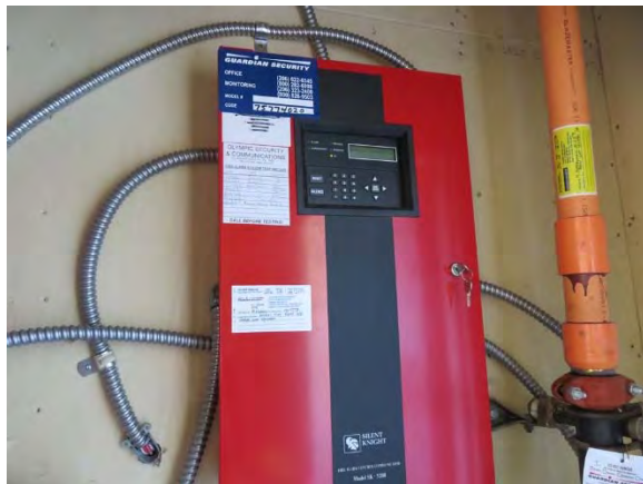
Typical Fire Alarm Panel
