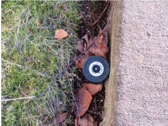
Typical Irrigation Sprinkler
